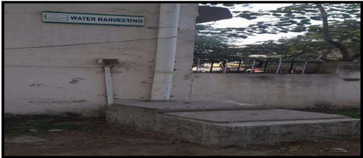
Rain water harvesting building back sides
