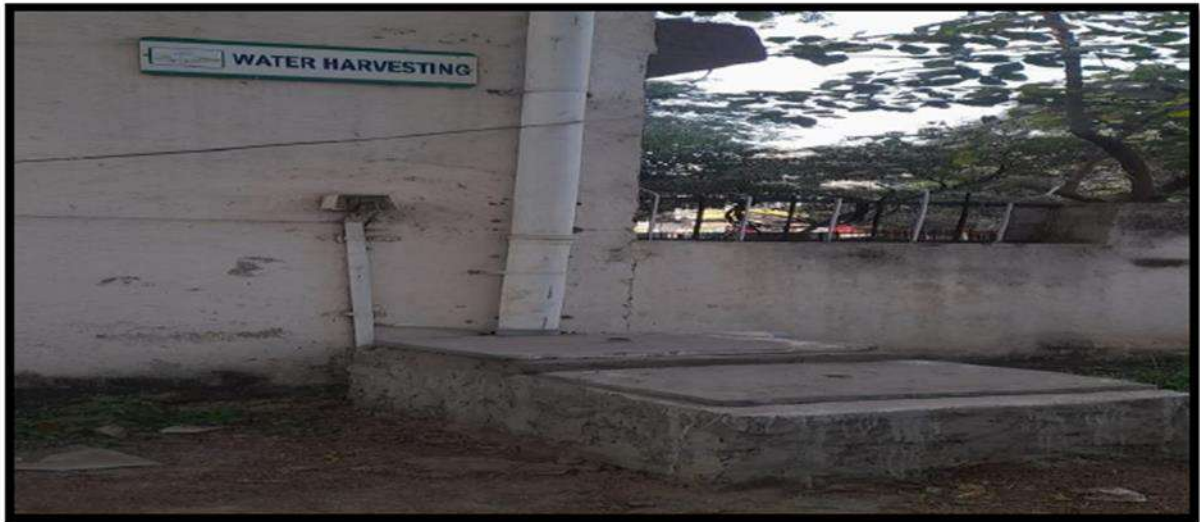
Rain water harvesting building back sides
