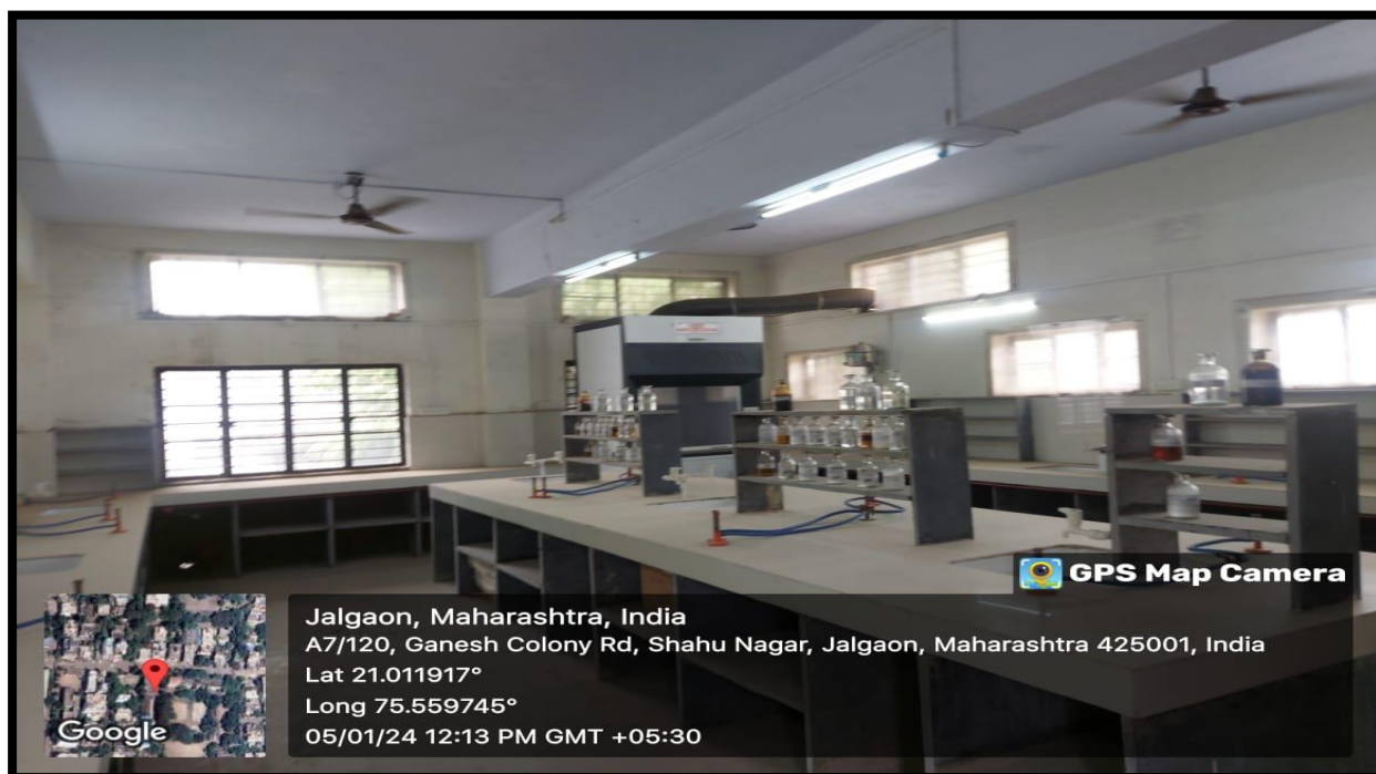
LED Tubelights in Chemistry Lab Main Building Campus
