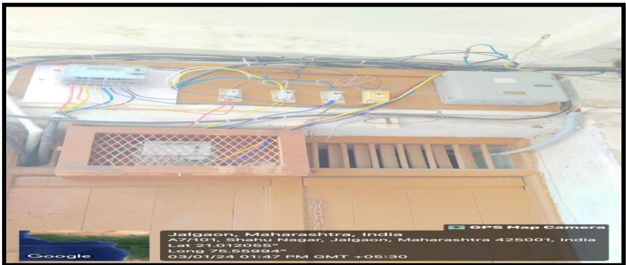
Solar plant Meter
