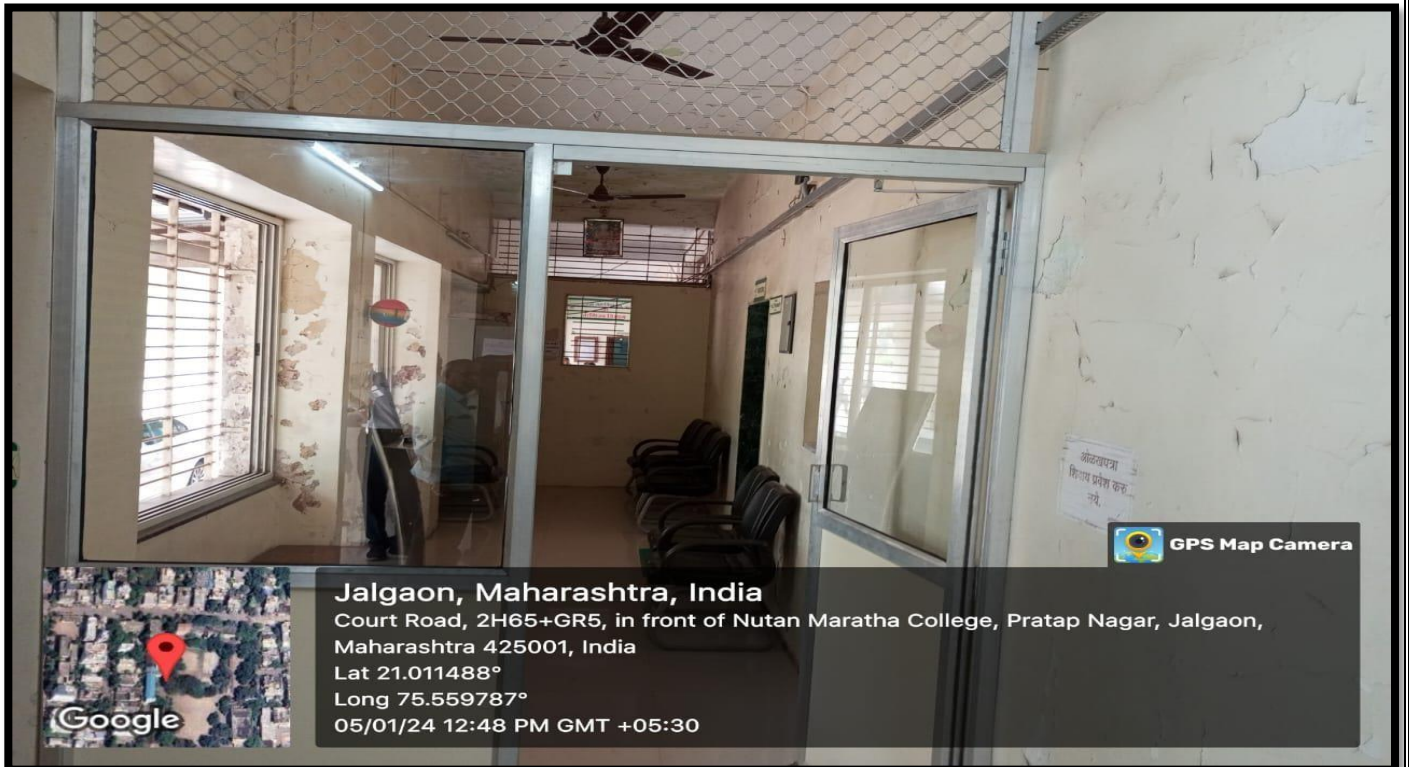
LED Tube lights in the Waiting Room outside Principle Cabin
